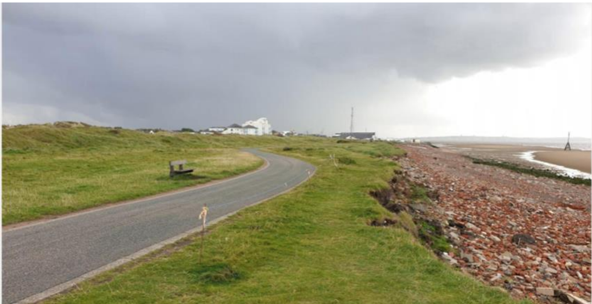
Eroding coastline at Crosby adjacent to the path
